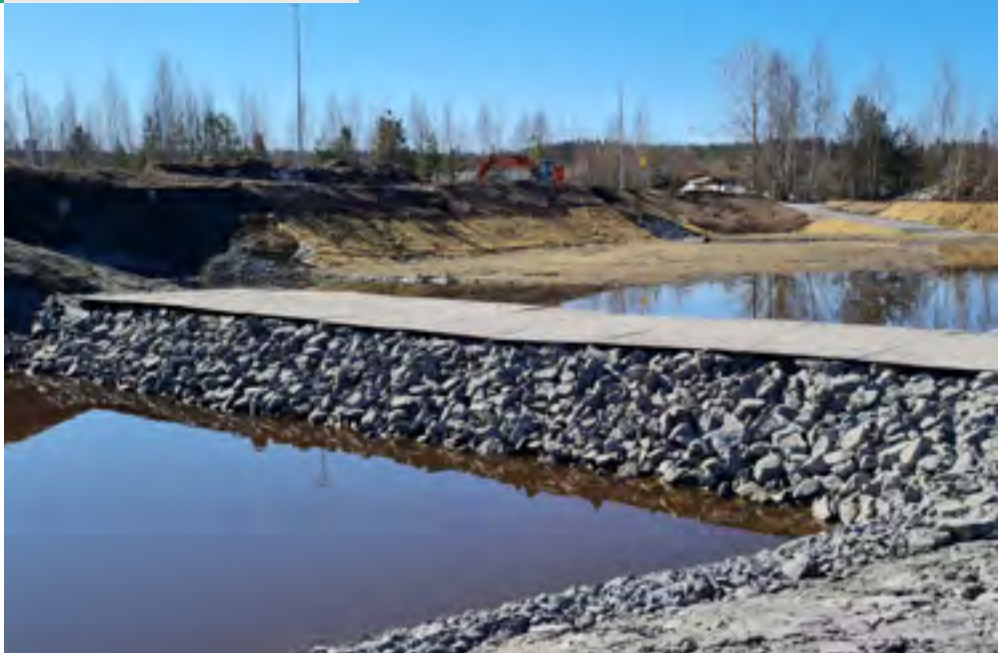
Completed dam filters water before discharge.
