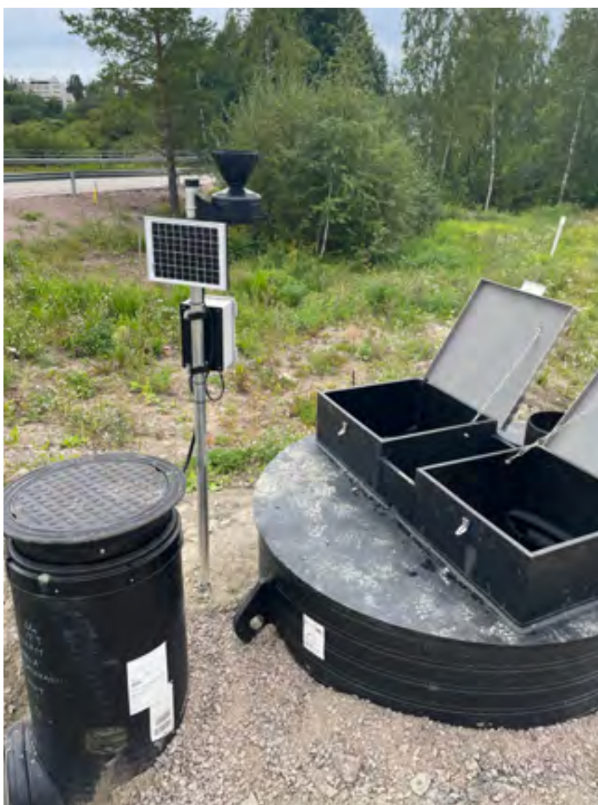
Filter chamber combines sedimentation and Filtralite P filtration.
